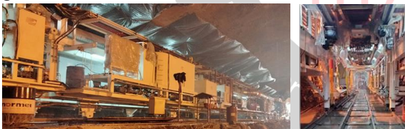
Figure 5. TBM Backup System
